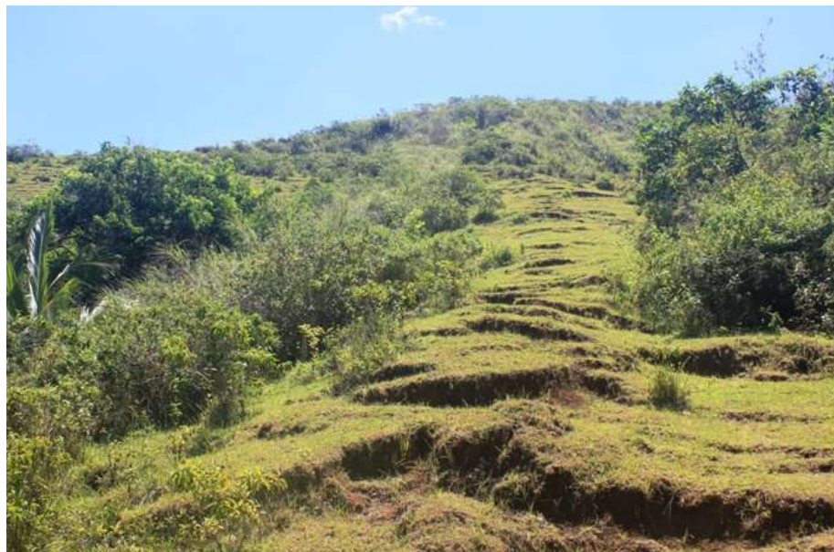
Figure 6. Erosion rills and cracks across the slope are common in several slopes of the marginal upland
